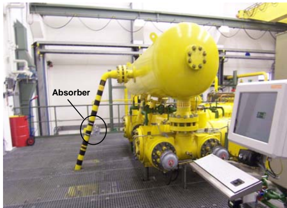
Figure 10: Photograph of the installed three-dimensional vibration absorber
