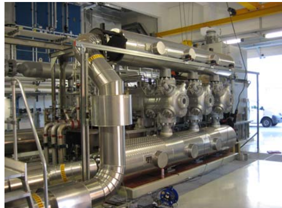
Figure 13: 1 st stage of the 6-cylinder reciprocating compressor plant with VFD-driven e-motor drive
